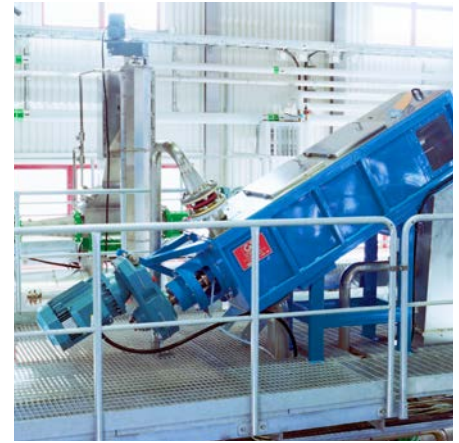
Thickening by inclined screw dewatering.
